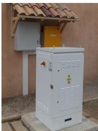
Figure 1- Battery installed at customer premises
