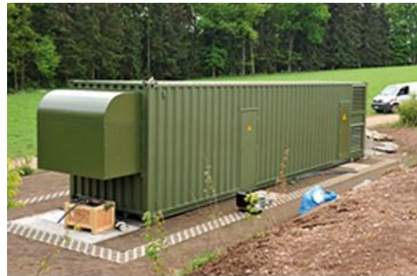
Figure 2: Active Voltage Regulator at MV
