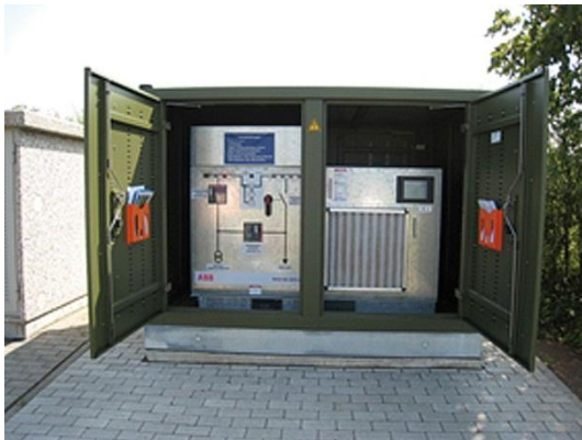
Figure 1: Active Voltage Regulator at LV
